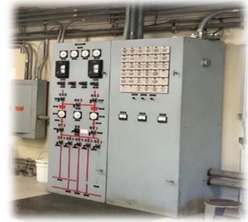
Main Breaker Panel
